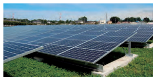
Tsurugashima Photovoltaic Power Plant (Tsurugashima-shi, Saitama Prefecture)
