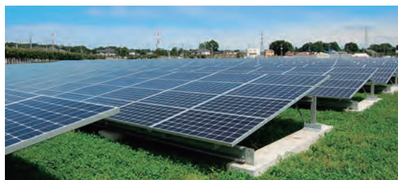
Tsurugashima Photovoltaic Power Plant
